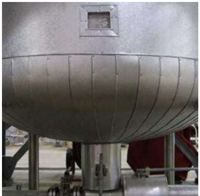
Tank head insulation for heat conservation
