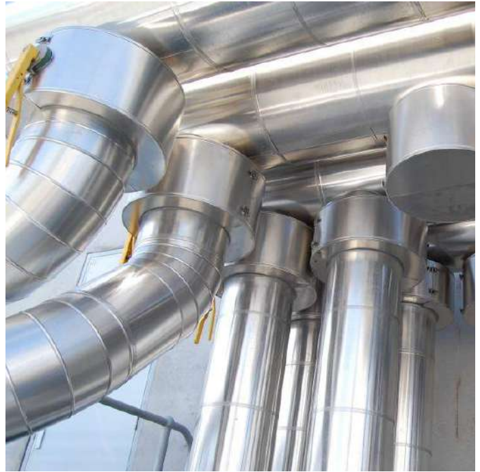
Hot insulation for pipeline
