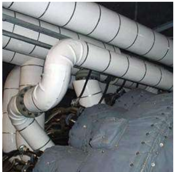
Hot insulation with non metallic cladding
