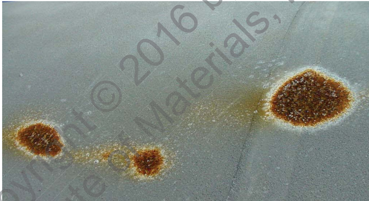
Figure 4 Premature coatings failure
