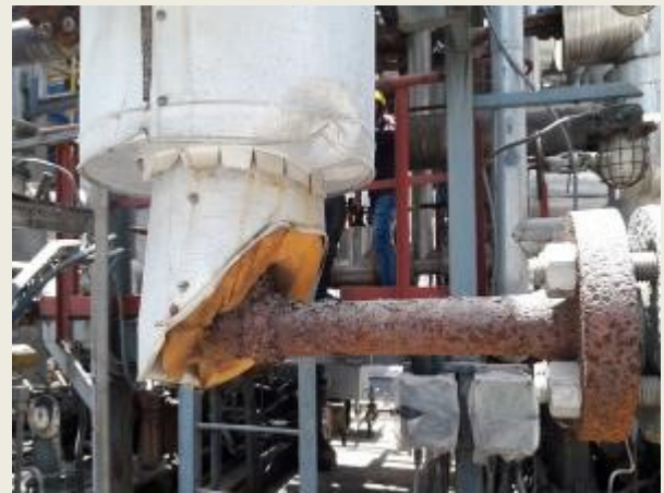
Figure 3: Badly installed and maintained insulation system with serious CUI
