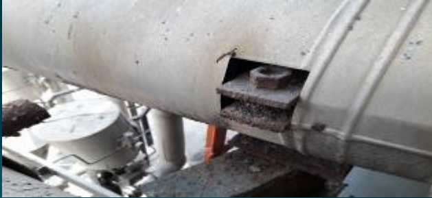
Figure 1: Poorly executed insulation installation at the support of the pipe.
