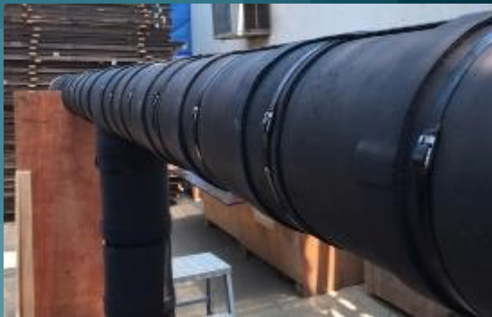
Figure 2: Carefully designed and installed insulation ensure the integrity of the system to deliver its functions.
