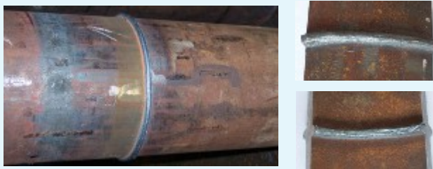
Figure 1: Pipe welded joint of OD168 x 7mm pipes of steel X70 and flash formation
