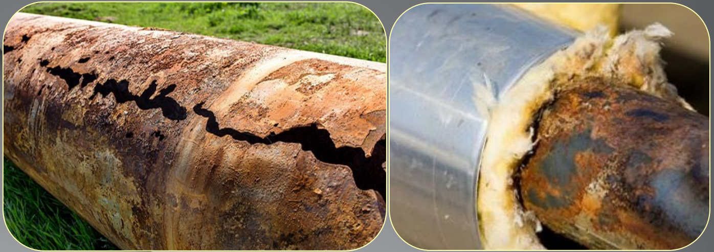
Figure 2: Corrosion in pipelines which results in economic loss and environmental pollution.
