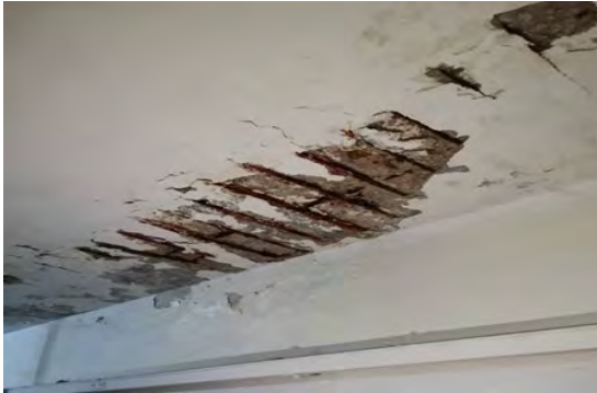
Figure 8 Spalled concrete under the soffits
