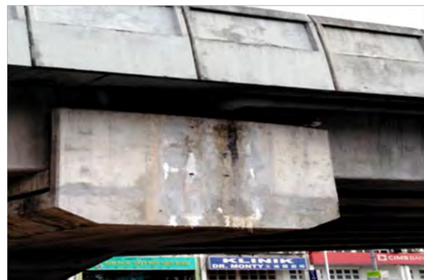
Figure 5 Calthemite on a concrete bridge
