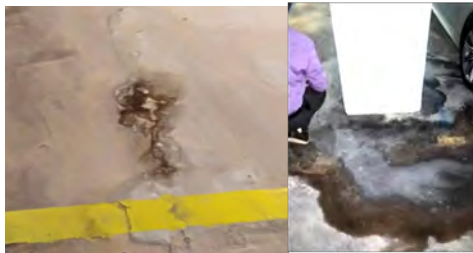
Figure 12 Rising ground water
