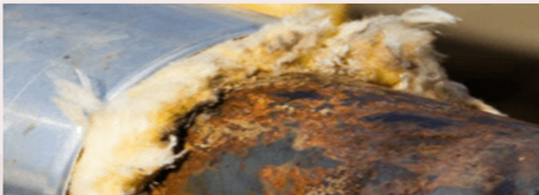
Figure 1: Corrosion of insulated pipe due to Wet Insulation contribution to Corrosion Under Insulation.
