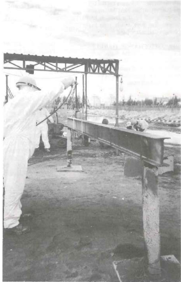
(Photo courtesy of Bredero Price - Kuantan, Training of IMM-CORAL Protective Coatings Technician Training & Certification Scheme)
