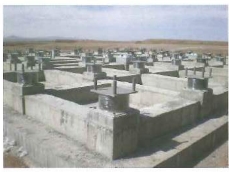
A complete installation of seismic rubber bearings for one of the buildings
