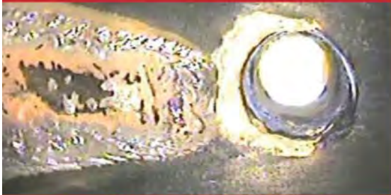
Internal Corrosion of Pipeline
