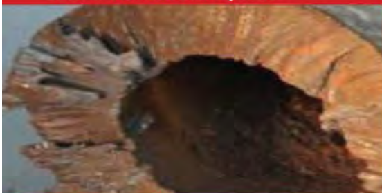
Pipe Crack Failure
